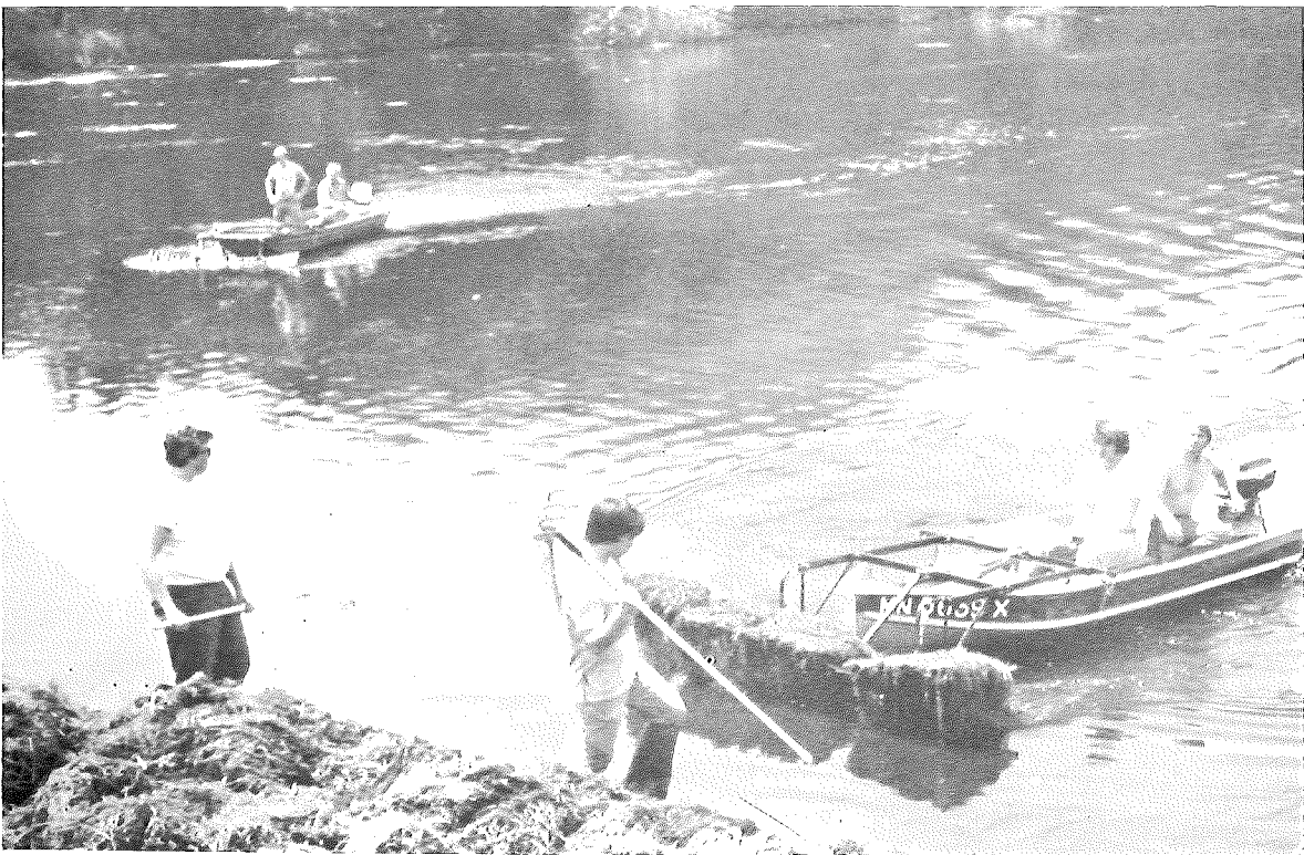
Figure 9-7. Above: City employee operating a Hockney C-10 weed cutter. Below: City crew using Air Lec WR-30 weed rakes to gather cut weeds.
