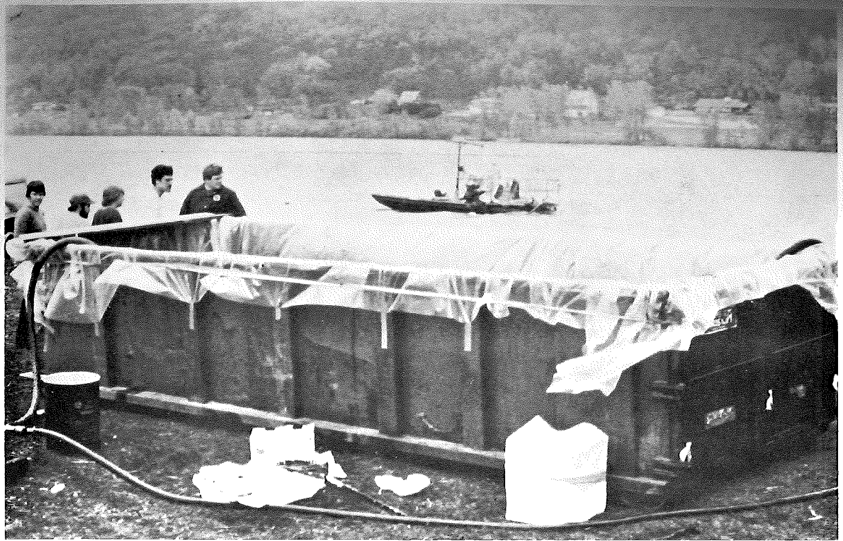
Figure 15-4. Heavily-weighted SCUBA divers with dry suits used hoses to remove heavy density oil from the lake bottom. The oil was sucked upward by a pump on a pontoon boat and piped to a temporary storage container on shore.
